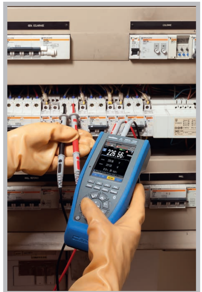
Measurements on electrical cabinets
